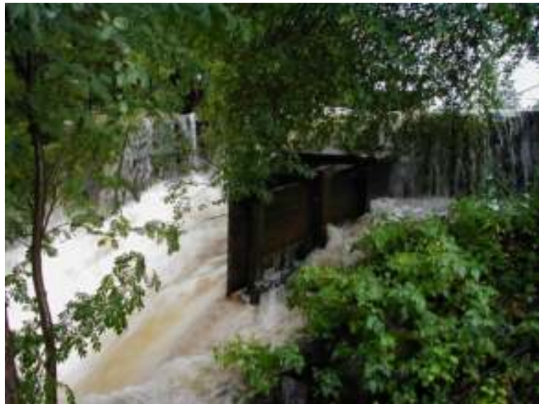
Image 3. Sidsjö Dam after extreme rain in August 2001.
